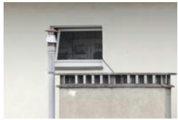
Power cable reaching the socket
