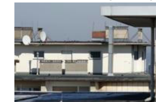
Power cable on the roof
