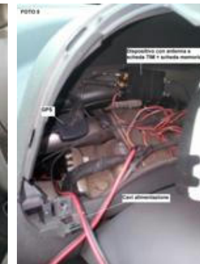
Counterclockwise from top: device with antenna, SIM and memory card; GPS; power cables
