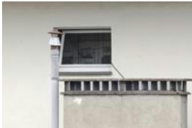
Power cable reaching the socket
