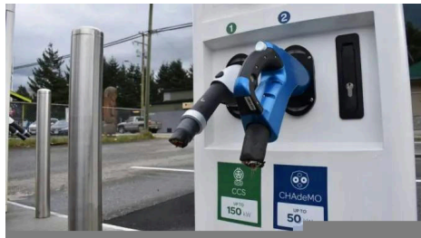
Electric vehicle charging station with severed cables.
