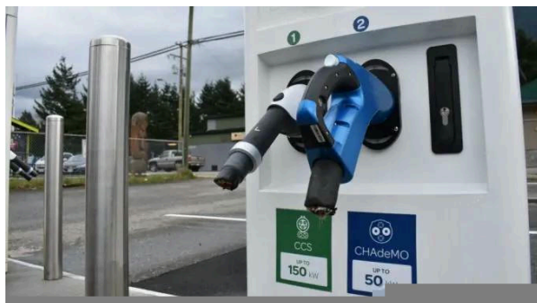
Electric vehicle charging station with severed cables.
