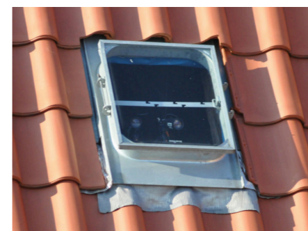
A camera found in the skylight of a public school in Berlin, Germany, in July 2011 22 .
