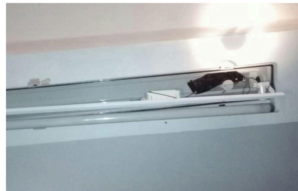
A microphone found inside a neon ceiling light in Modena, Italy, in December 2015 6 .
