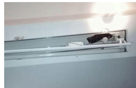
A microphone found inside a neon ceiling light in Modena, Italy, in December 2015 15 .
